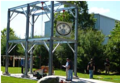
Pipefitters Local 537 want to construct a rigging structure similar to one constructed by their sister local, Pipefitters Local 51 in Rhode Island
