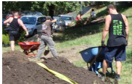
From the left Travis Stewart, Karen Chaffee and Desmond Rohan build the Rain Garden. In the background Janice Geary and John Lowe install erosion preventing netting over newly planted small native shrubs.
